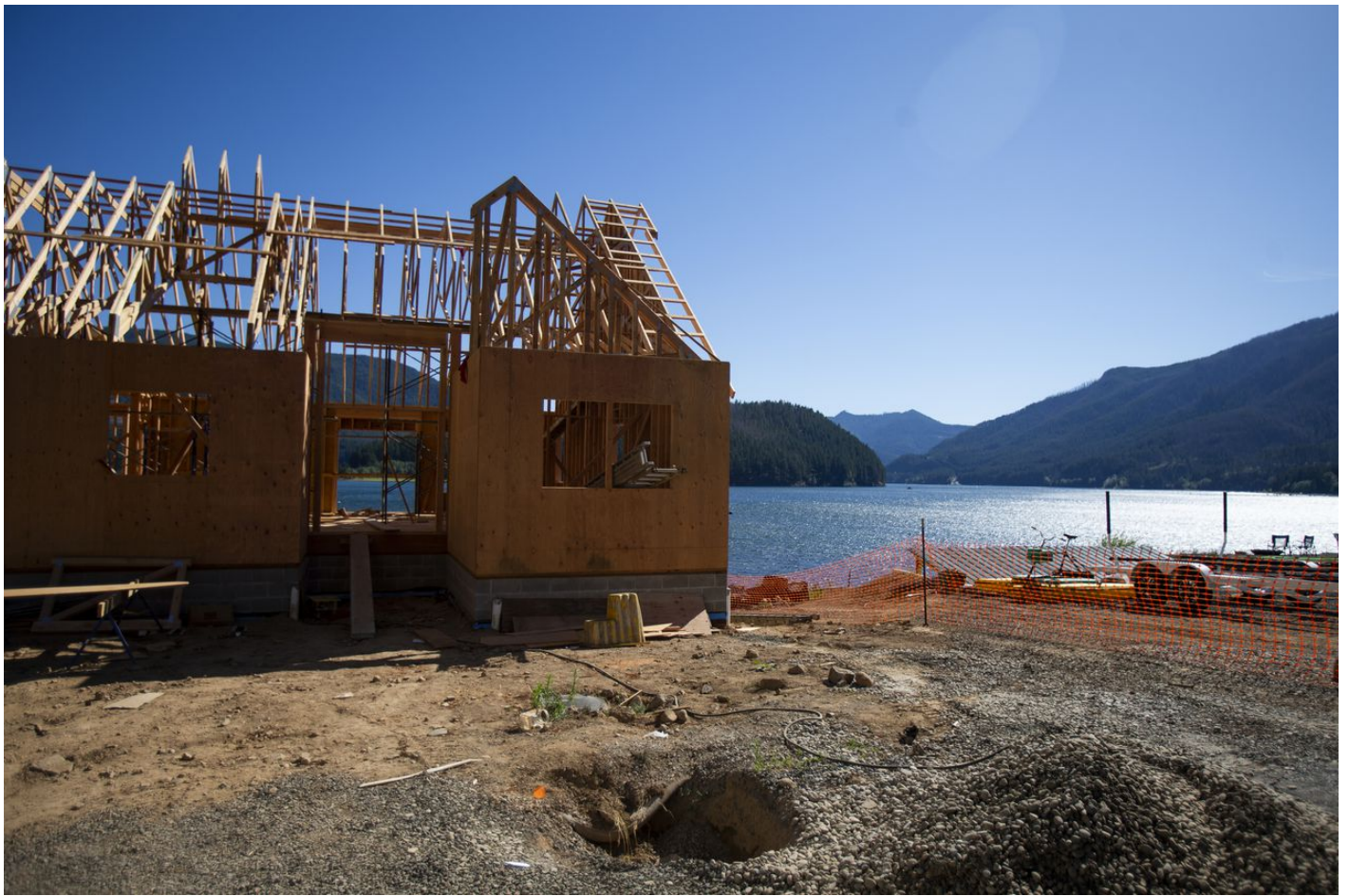
A house under construction in Detroit, Oregon, on Friday, July 22, 2022. Many of the structures in Detroit were lost to the Beachie Creek fire in the summer of 2020. Some residents of the Santiam Canyon who lost their homes in the fires of 2020 are still going through the rebuilding process two years later. Dave Killen / The Oregonian
